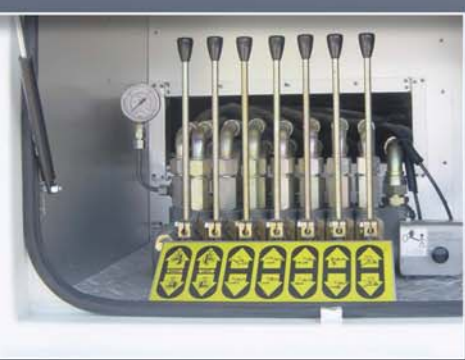
KUMANDO PANOSU CONTROL PANEL FOR ALL HYDRAULIC INSTALLATION
